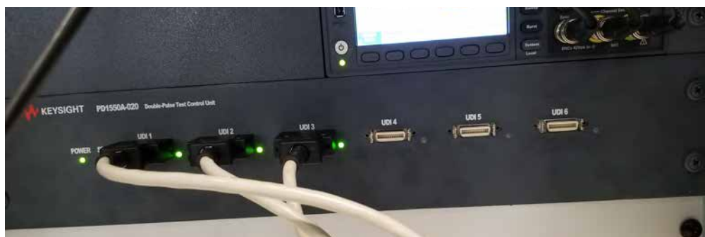
Figure 33 UDI Cables Connected to Control Unit Front Panel
